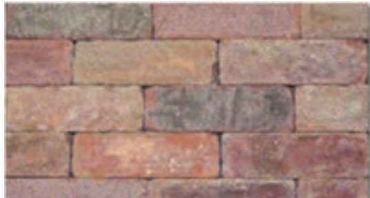
No Mortar Joint (Dry-Stacked)
