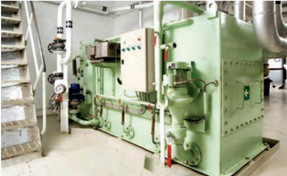
sewage treatment plant
